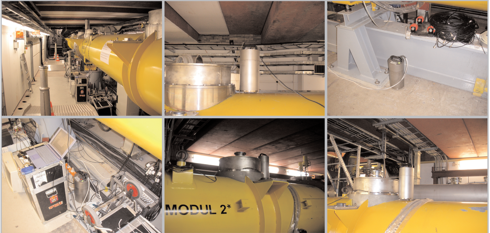
View of vibration measurements on the floor and on the module 4 and 2* at TTF.
