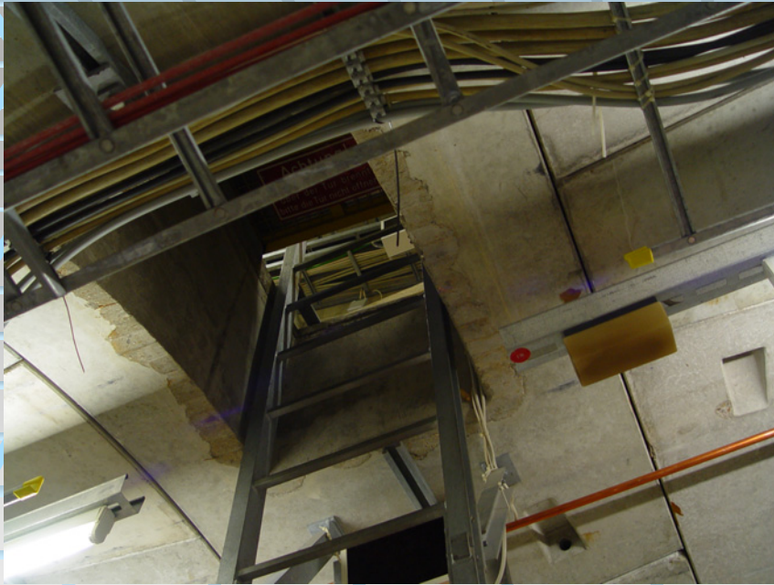
PETRA-HERA injection point (WR217)
